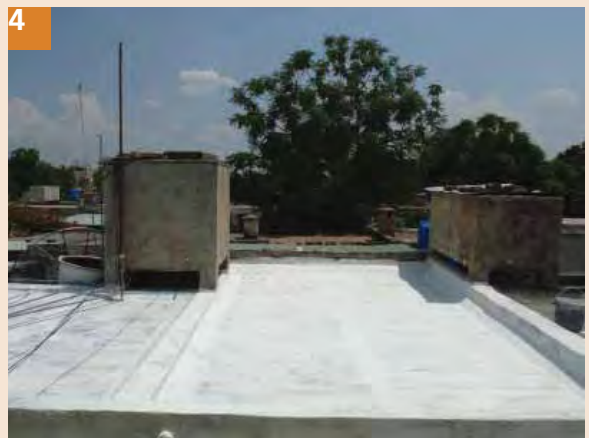
4 Rubber paint should be thoroughly applied in all corners and wall junctions to avoid leakages from all parts of the slab and let the surface dry for one day.
