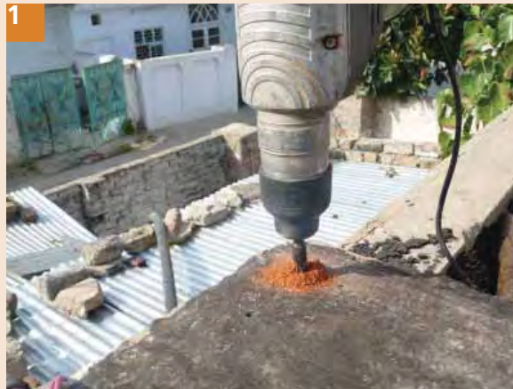
1 Drill holes in slab on corners to fix MS bed plate. Care should be taken while working near the corners to avoid falling down. Manual drill can also be used if electric drill is not available.
