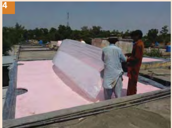
4 Cover the foam (extruded polystyrene) with another plastic sheet in order to protect its surface from fresh concrete and water. Cut 1 ft diameter semicircles in the foam to allow drainage at spouts.
