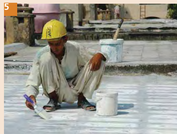
5 Use two coats of white appoxi on top surface to improve performance of slab by reflection and to enhance water proofing properties.
