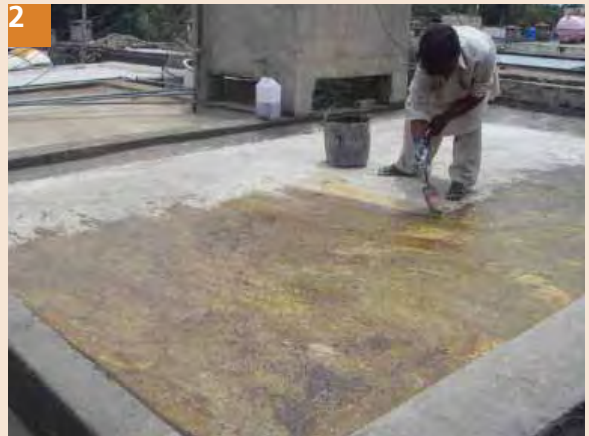
2 Apply 1st coat of AC cleaner to remove existing chemicals and dust from the surface. AC cleaner is used to remove chemical impurities particularly.
