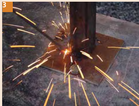
3 Weld MS square conduit pipe of 1-1/4 inch size vertically for framing. Use safety lenses during welding. Provide proper and continuous welding layer for strength and durability.
