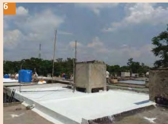
6 Apply final coat of Rubber approxi of OCEVA-MOL mixed with white cement and let the surface dry for two days.
