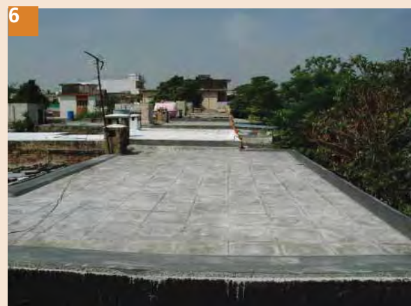
6 Cure the surface for a minimum 3 days period. Lime wash can be used above to make it reflective and improve the performance of tiles.
