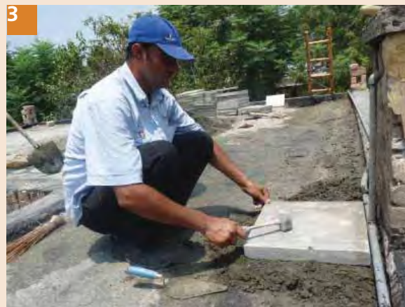
3 Lay and fix the tiles starting from the edges. Use rubber hammer to avoid damage to the tiles and to ensure tiles are properly set and fixed in mortar.
