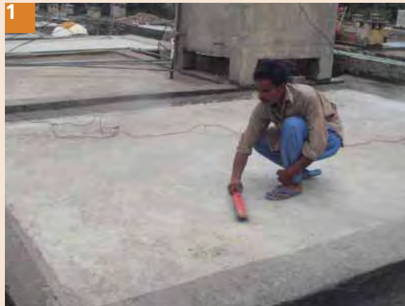
1 Clear the surface, use grinder to remove all marks and sticking material from the pours of concrete.
