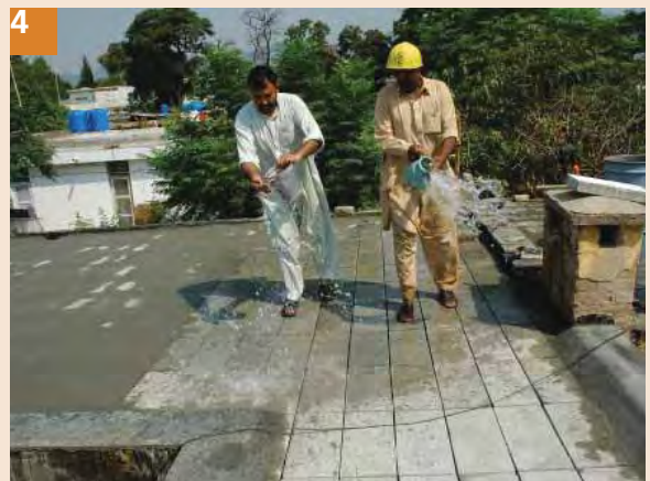
4 Cure the tiles before providing cement slurry on the top so that tiles may not absorb water from the slurry.
