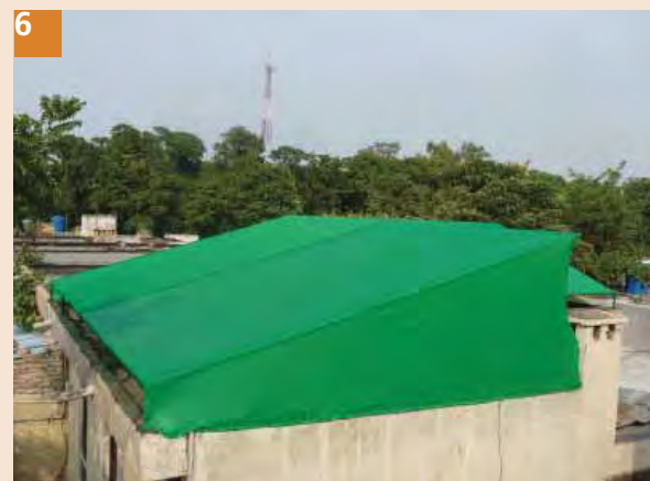
6 Make the frame and fix net in such a way that access would be possible on the roof, openings on both sides will help cross ventilation
