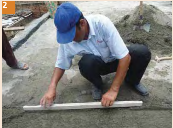
2 Fix tiles in cement sand mortar (1:4), mortar thickness is 1 inch, use mortar within 45 minutes of addition of water to it. Thickness of mortar should be kept constant throughout the slab.
