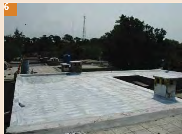
6 Surface needs to be cleaned frequently to maintain good reflective shine.
