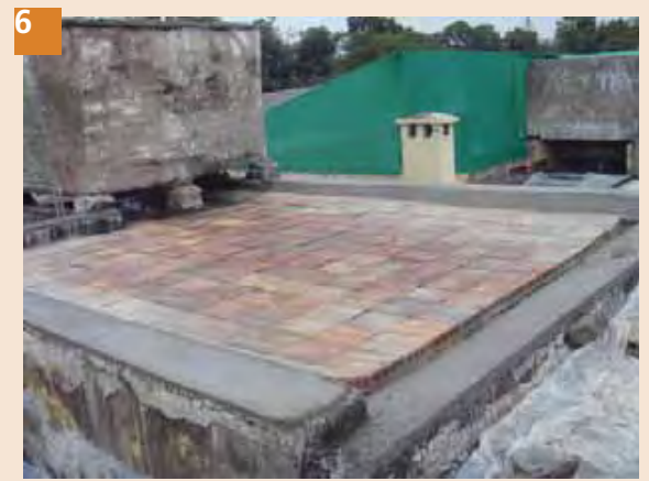
6 Cement sand mortar should be cured for at least three days to ensure proper setting of cement.
