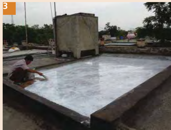
3 Let the surface dry after using AC cleaner for minimum 6 hours. Provide first coat of OCEVA-MOL liquid rubber.
