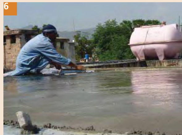
6 Cover the whole roof with 2 inch thick concrete 1: 2: 4 (cement:sand:aggregate) and level the concrete surface with float. The concrete will provide a wearing coat and protect the foam.
