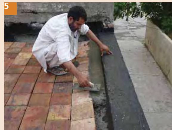
5 Fix the tiles from sides/edges with the help of cement sand mortar (1:4) so that tiles could not be displaced easily.
