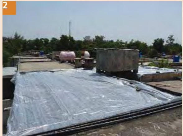
2 Cover the roof with plastic sheet (1/2 mm polythene). The plastic sheet should cover the entire roof and edges.
