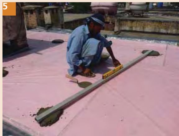
5 Maintain the same slope for the concrete for drainage as per slope of roof slab.
