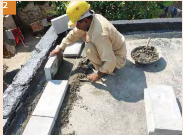
2 Lay the tiles starting from the edges in cement sand mortar (1:4). Use rubber hammer to set the tiles to avoid any damages. Mortar prepared should be used within 45 minutes of addition of water.
