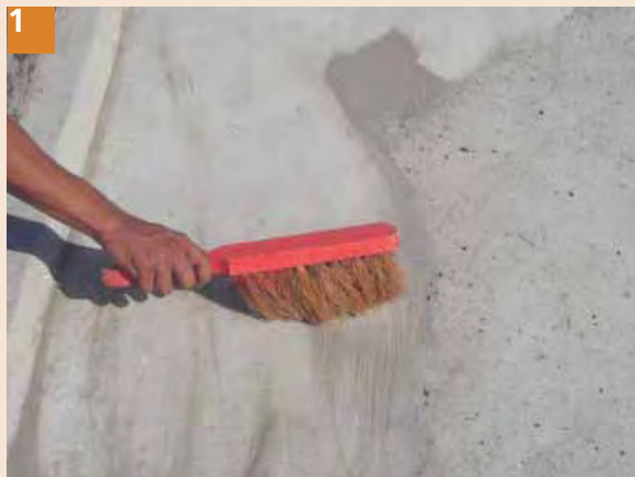
1 Use coconut brush for proper cleaning and removal of dust from the roof.
