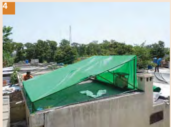
4 After fixing the frame, fix green net. Remove wrinkles by tightening. Use copper wire to fix the net, care should be taken to avoid tearing of net.
