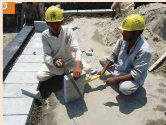
3 Use hand saw to cut the tiles if electric tile cutter is not available. Cover the entire roof with tiles and leave no space empty.
